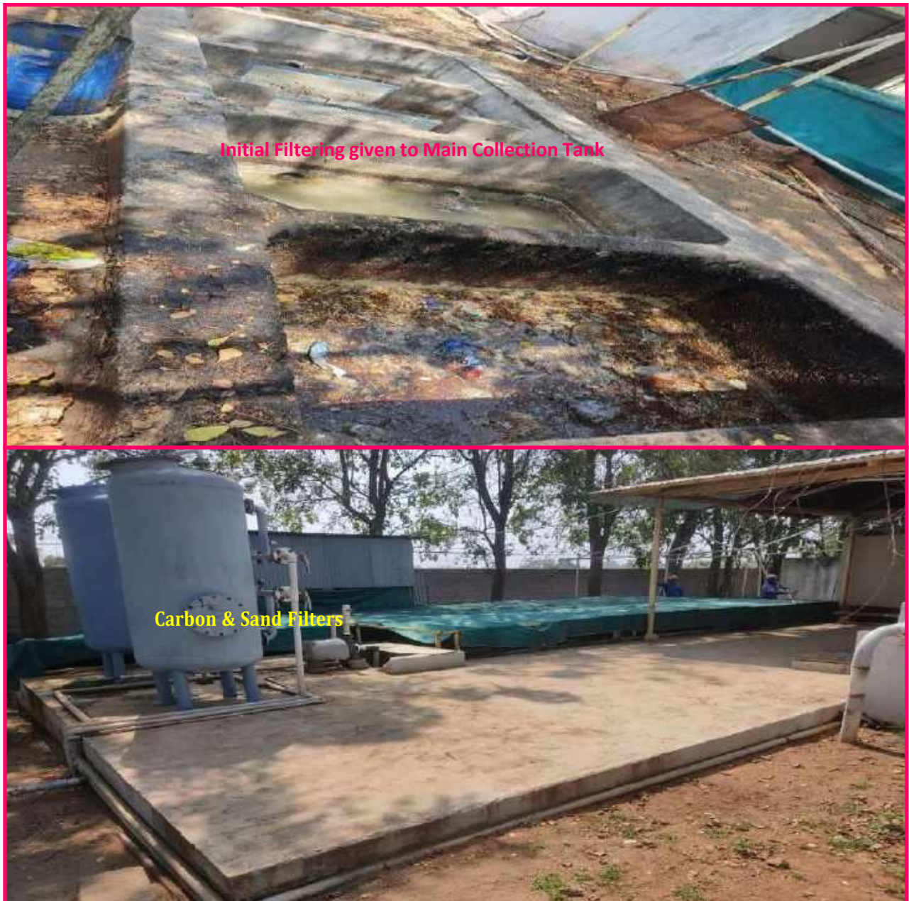
Fig.3: Snap shots of Sewage Treatment Plant (STP)
