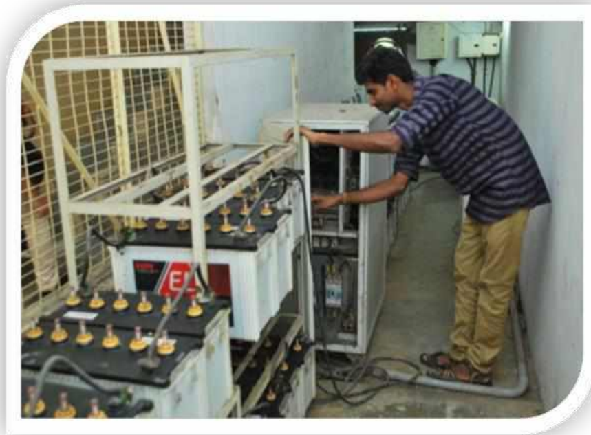
Figure B. 6.2c Servicing UPS Equipment
