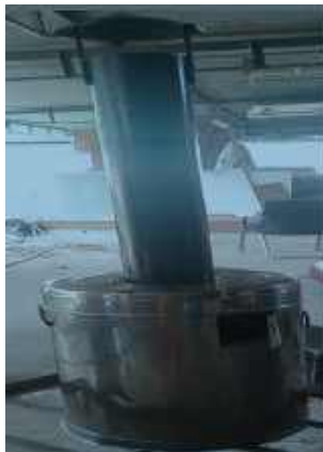
FIGURE B 9.4.3k Incinerator for Bio-Degradable Waste
