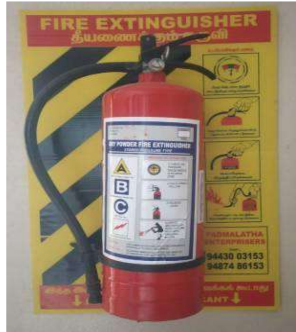
Figure B. 6.3f Fire extinguisher in all laboratories
