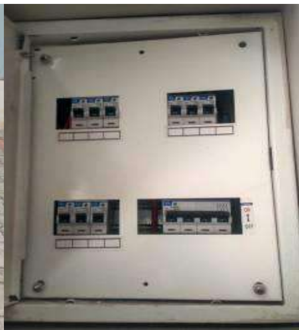
Figure B. 6.3h Electrical Wires Protected by RCBO and Fuses in laboratories
