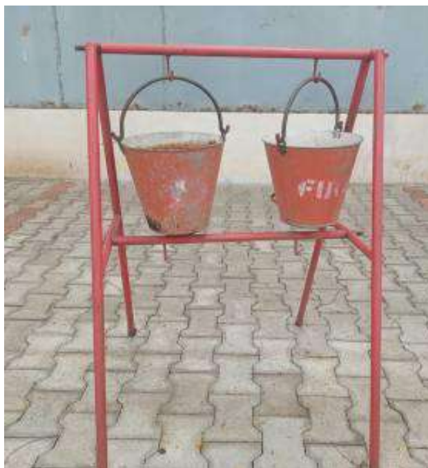
Figure B. 6.3g Fire accident prevention buckets near laboratories
