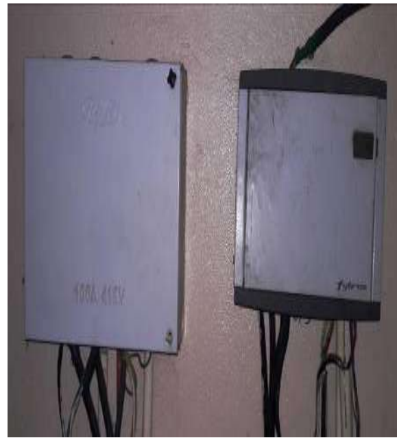
Figure B. 6.3d Electrical Wires Protected by MCB in laboratories
