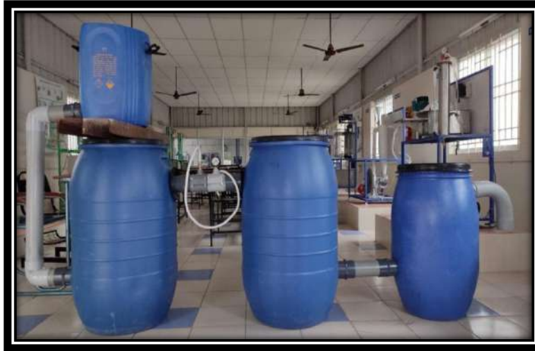
FIGURE B 9.4.3i Automation in Bio-Gas Plant
